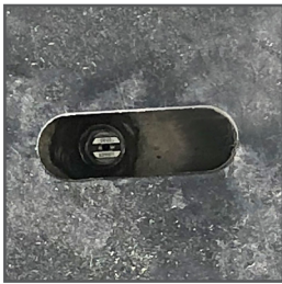
Twelve 15°, size 20 nozzles spaced 6-inches apart
